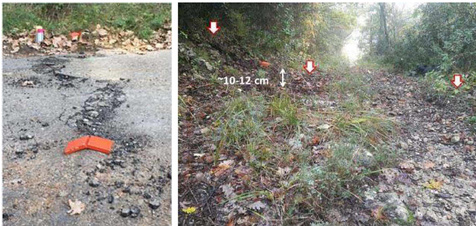
Figure 6. Examples of surface rupture evidences associated with the November 11, 2019 Le Teil earthquake (left: Northeastward view of en-échelon folds in an asphalt road associated with a slight uplift of the southeastern compartment; right: Southeastward view of 10 cm-high NNE-SSW trending fault scarp observed within a walking path).
