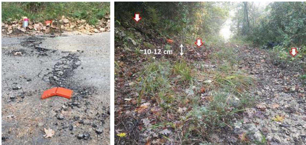
Figure 6. Examples of surface rupture evidences associated with the November 11, 2019 Le Teil earthquake (left: Northeastward view of en-échelon folds in an asphalt road associated with a slight uplift of the southeastern compartment; right: Southeastward view of 10 cm-high NNE-SSW trending fault scarp observed within a walking path).
