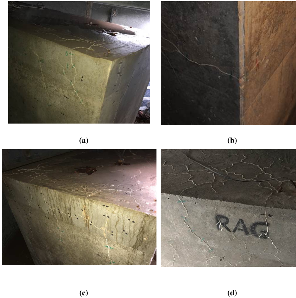
Figure 22 : (a) DEF mock-up at t = 537 days (b) DEF mock-up at t = 537 days (c) ASR mock-up at t = 512 days (d) ASR mock-up at t = 516 days
