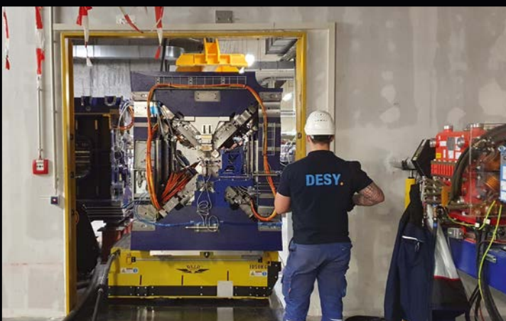
Figure 1: Transport of one of the APPLE-X undulators into the European XFEL undulator tunnel
