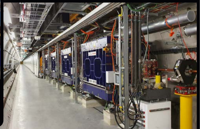
Figure 2: Four new APPLE-X undulator segments installed at the end of the SASE3 undulator
